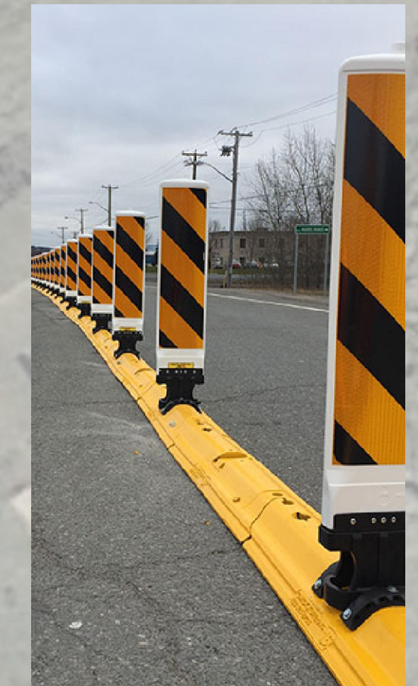
PHASE 1 - INSTALLATION OF QUICK KURBS AT MIDDLE SCHOOL NORTH SIDE CROSSING ON US-12. PHASE 2 WOULD INSTALL PERMANENT CURB WITH MDT APPROVAL AFTER TRIAL PERIOD.
