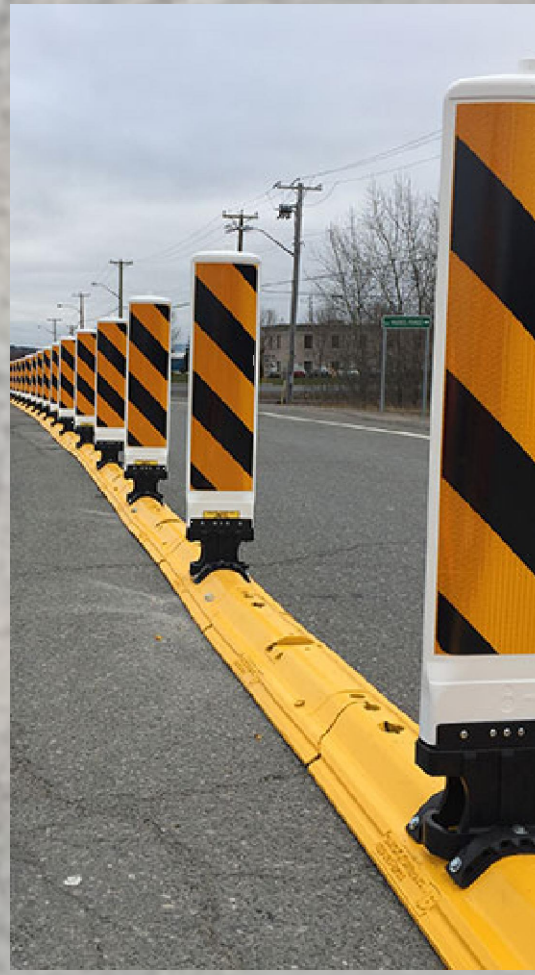
PHASE 1 - INSTALLATION OF QWICK KURBS AT TRAIL CROSSING ON US-12. PHASE 2 WOULD INSTALL PERMANENT CURB WITH MDT APPROVAL AFTER TRIAL PERIOD.
